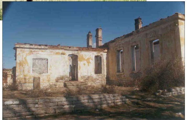
The remains of the main public library in the municipality of Malishevë (Southwestern Kosovo), which was burned down July 1998.
