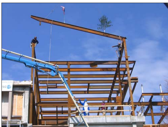
The structure for the new library building is completed in the "topping Off" ceremony
